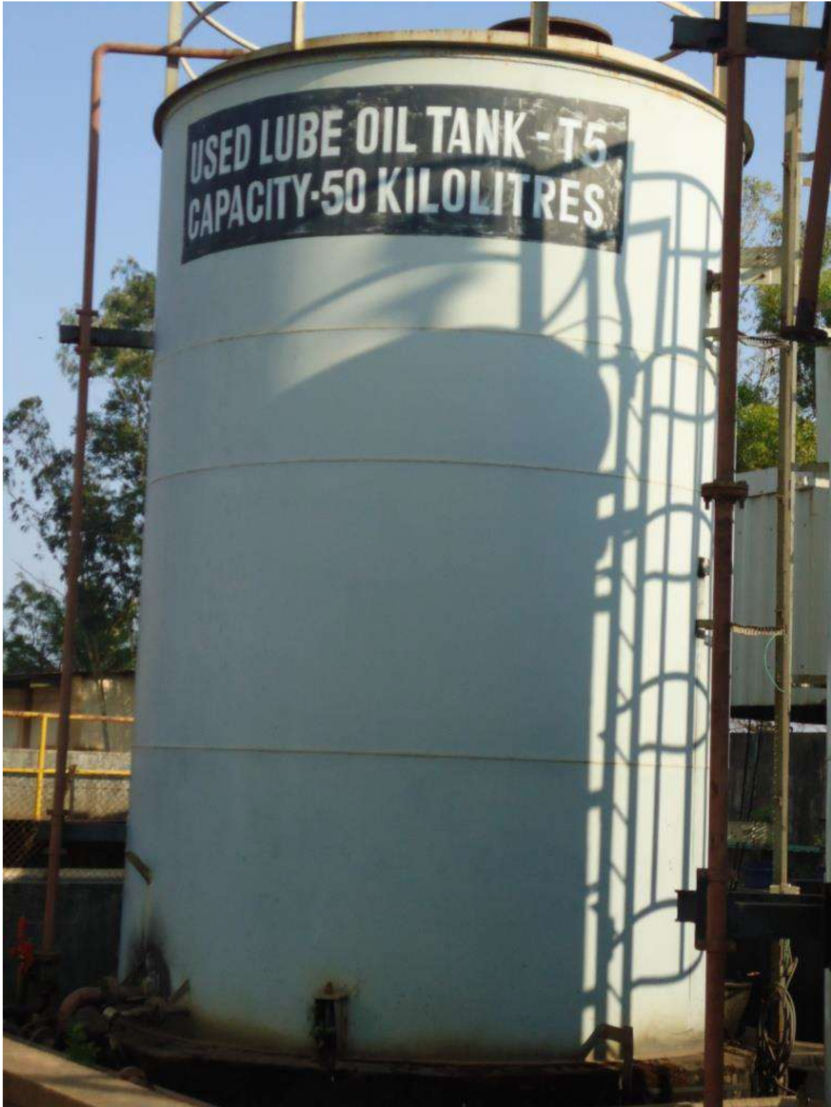
Oil storage tank
